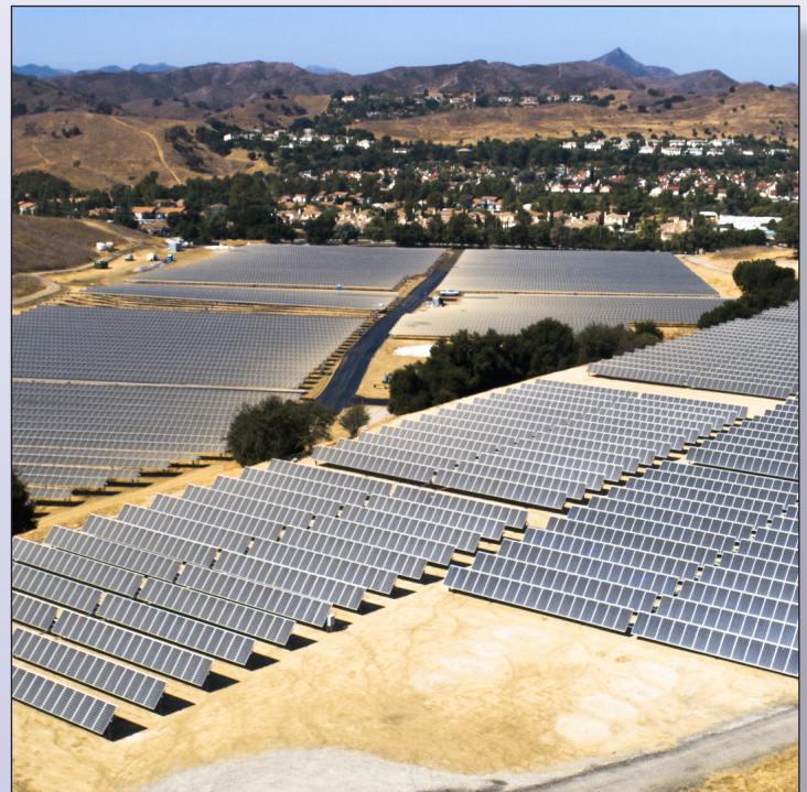
Five megawatt solar power facility used to offset the energy used by the Tapia Water Reclamation Facility
